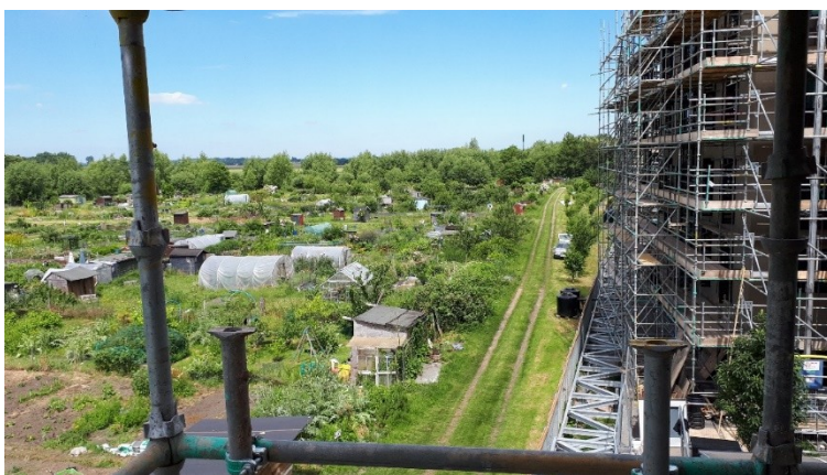
Works have progressed on 7 blocks with either scaffolding up or scaffolding down
